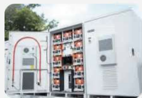
Energy storage container
